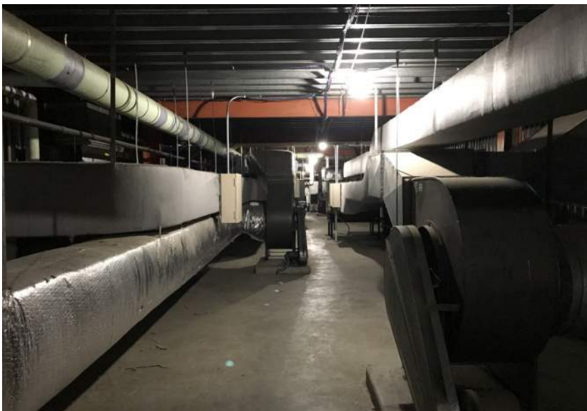
Interior Photo: Mechanical mezzanine
